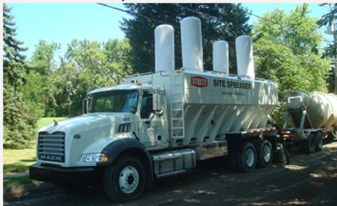
Spreader with popup filters on roof
